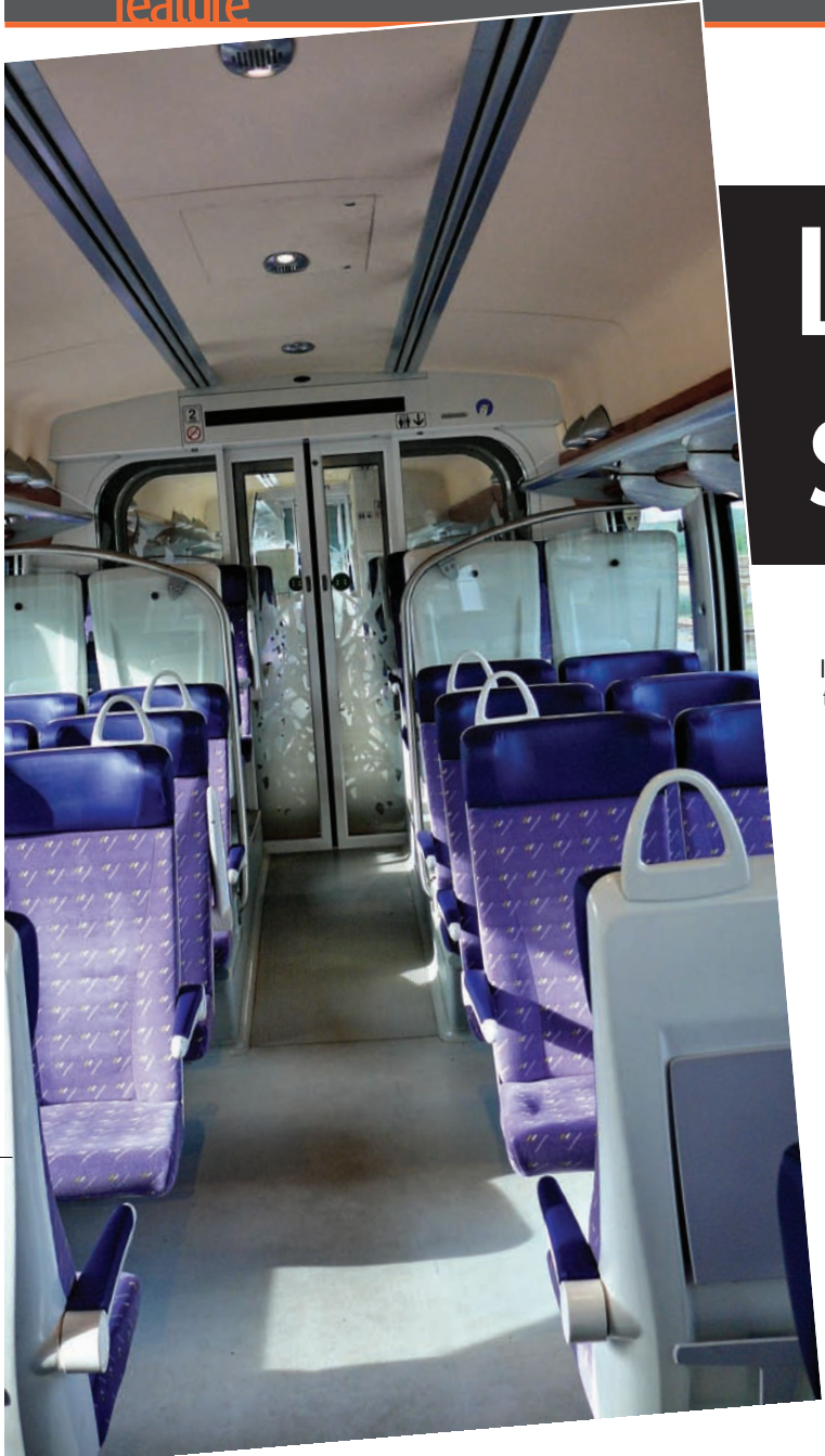
AGC train, fully illuminated with 154 LED reading lights and 85 LED down lights.
